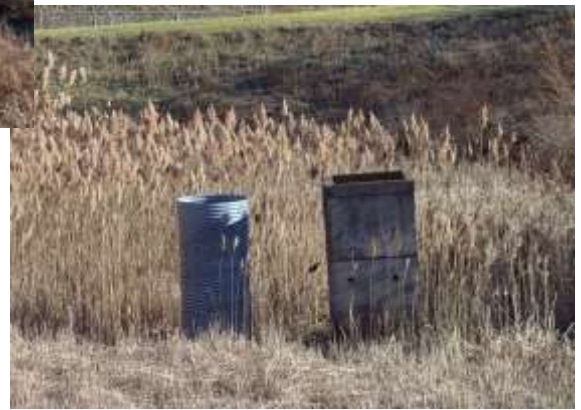
Overflow structures seen in the previous shot. Phragmites are in the back; other grasses in the front.
